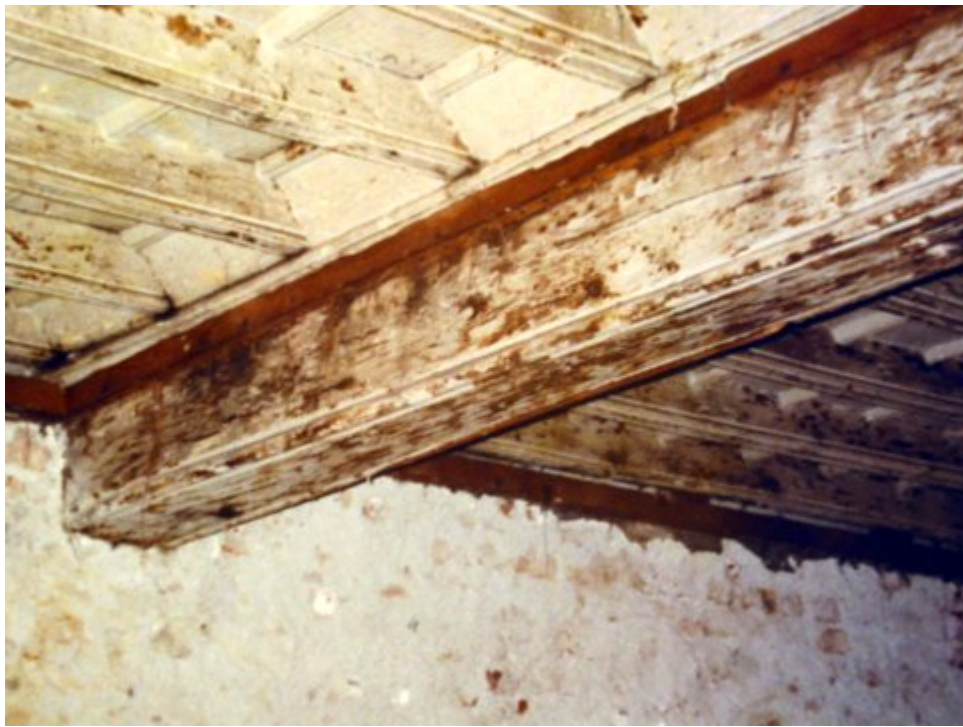
Figure 2.2: Comprehensive survey should be carried out before the strengthening of the old floor structure
