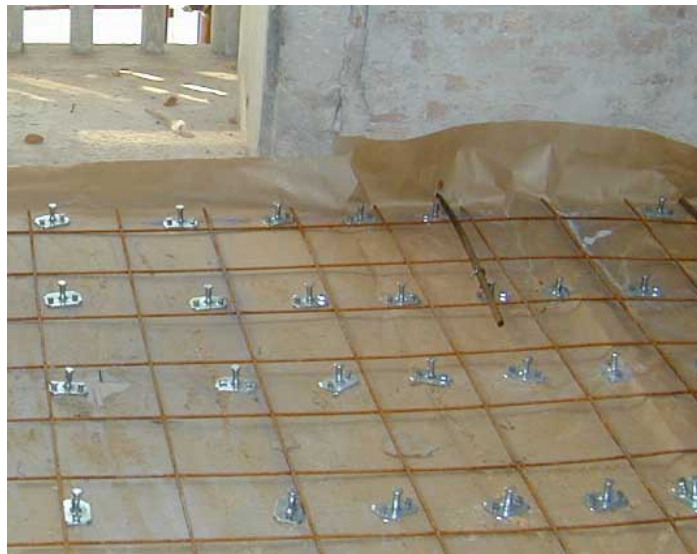
Figure 1.3: Before pouring of concrete it is necessary to put reinforcing mesh preventing development of cracks at the lower surface of a concrete slab
