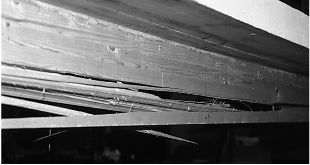
Figure 6.6: Typical failure of a timber-concrete composite beam: cracking of the timber beam due to tension
