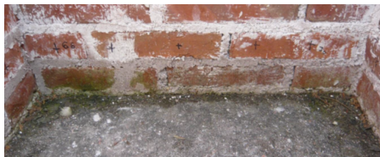
Figure 6.2: Bottom part of the wall after 13 months since its construction, water rising by capillary action, resulting in the growth of algae and lichen at the masonry surface.
