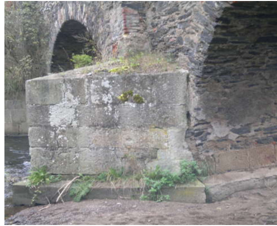
Figure 9: Weathering and biological growth on the central pier (Pudis a.s., 2015)
