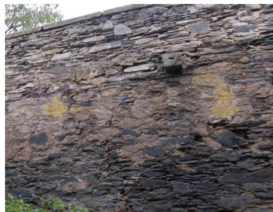
Figure 7: Weathering and plaster deterioration on the spandrel wall (Pudis a.s., 2015)
