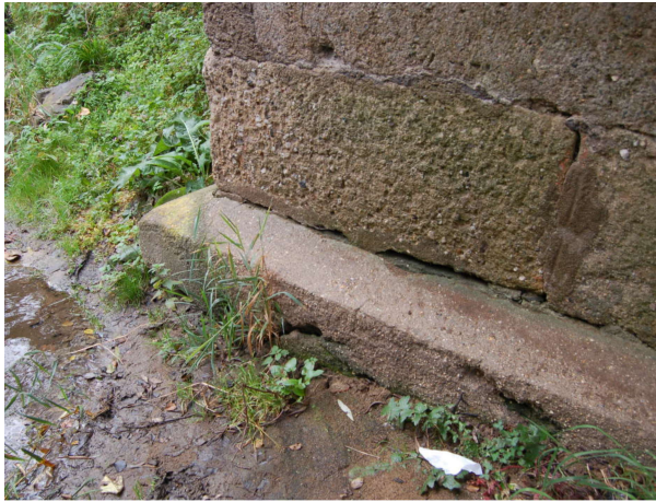
Figure 8: Weathering of pier materials (Pudis a.s., 2015)
