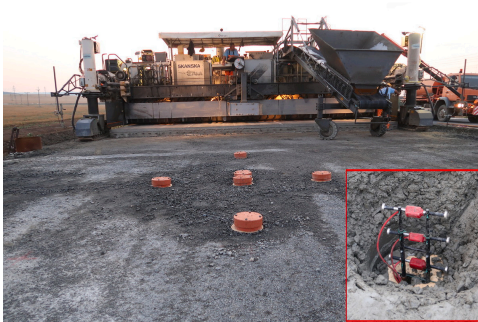
Fig. 3. Installation of the monitoring system. Prior to the casting, gauges were protected under the orange covers, assembled later to correct heights and filled back with concrete.
