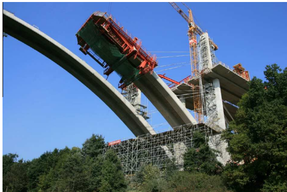
Fig. 12. Two arches of Oparno Bridge during construction (Photo by Jan L. Vitek).
